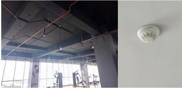
Gambar 4. Sprinkler, Heat detector, Smoke detector dan alarm.
