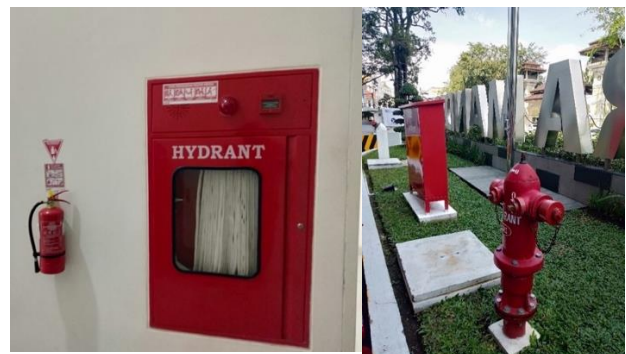
Gambar 2. Fire extinguishers dan hydrants.
